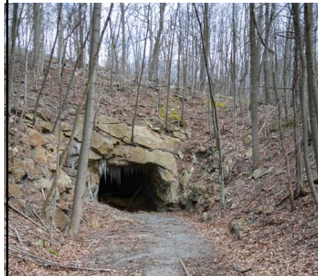
The south portal of the Sideling Hill Tunnel on the East Broad Top main line, which would only require "moderate" work to reopen, according to EBT Foundation General Manager Brad Esposito.
