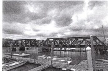
The India Point Railroad Bridge spanning the Seekonk River in 2022. (David L. Ryan/Globe Staff)
