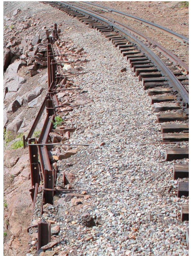
In this photo, you can see that the tracks and roadbed were held in place by old rails and metal hooks embedded in the side of the mountain. It’s a little bit terrifying in hindsight! (Note guardrail, also.-Ed.)
