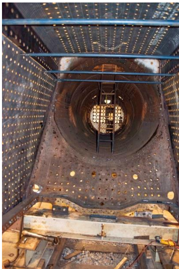
View through the fire door in the boiler backhead of No. 1361 shows the custom-fabricated side wrapper sheets, left and right, the Belpaire plates, upper left and upper right, and the roof sheet, top. The four horizontal stays are temporary to stabilize the components for fitting and welding. Dan Copper
